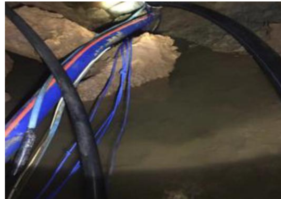
Pumping line inside the spring
