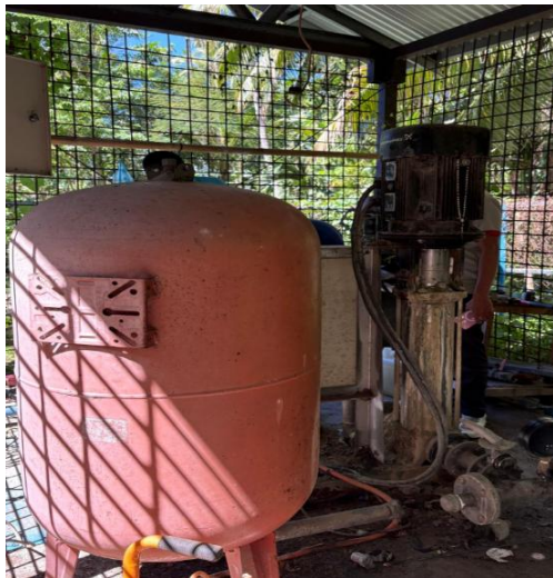
Existing water pumping system
