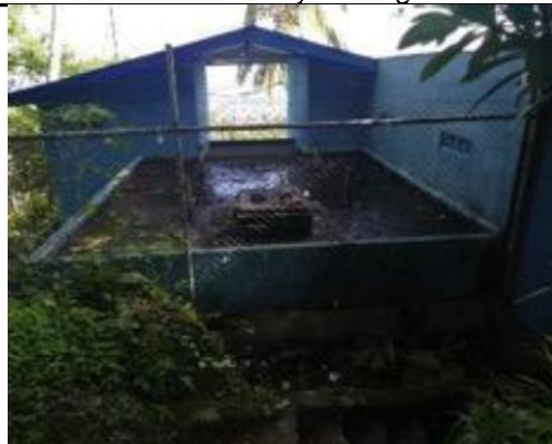
Current condition of the Lamegua tank where it's located 520 m SW towards the Opt. 2 location
